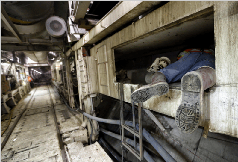
These miners sometimes have to get into tight spaces while working inside the tunnel boring machine.
